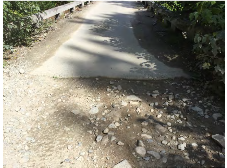
Potholes right approach
